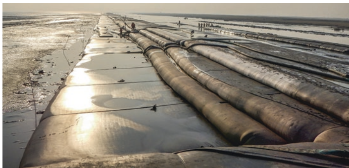
Fig. 31.2 A seawall is being built in the Yangtze River estuary (From Ma et al. 2014)
