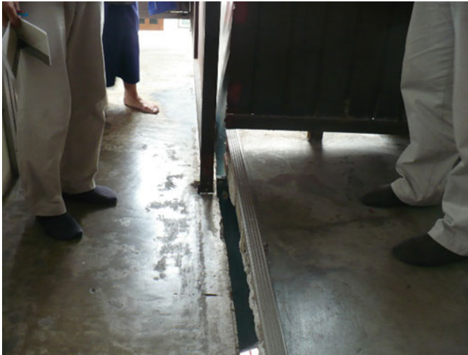
Fig. 8.14 A cracked building by land subsidence. Source Author's fieldwork (2009)
