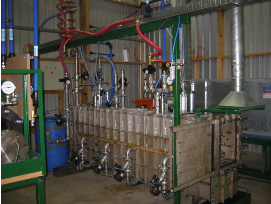
Plate 4 Unitreat pilot plant located at the University of Melbourne, Creswick
