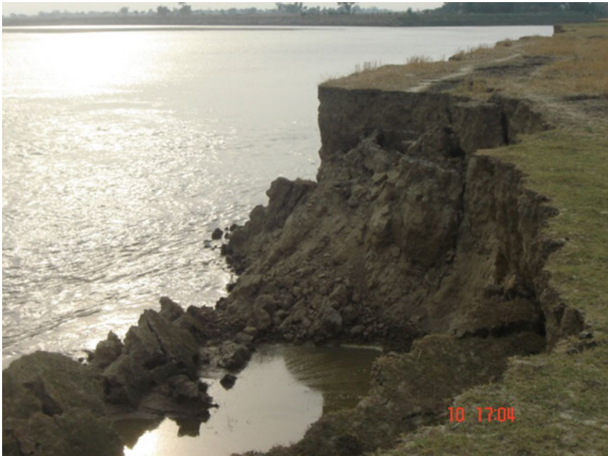
Fig. 15 Lateral erosion in Ghaghara River in Deoria district, Uttar Pradesh, Ganga Plain
