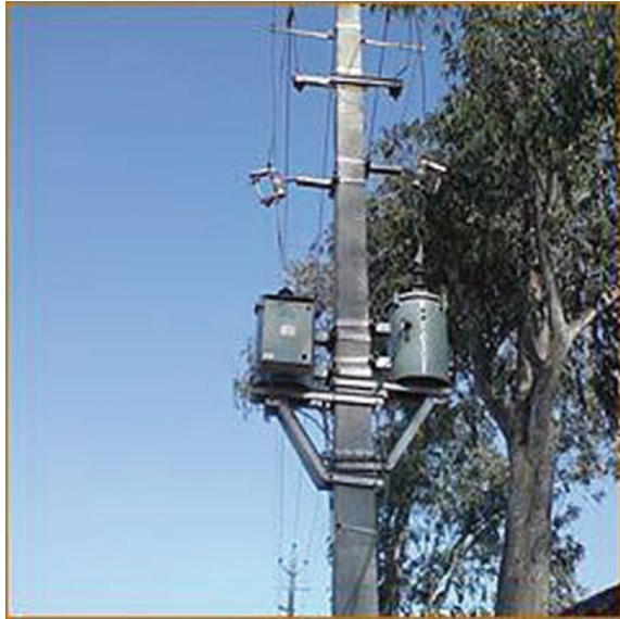
Fig. 7.1 HVDS used in rural electrification
