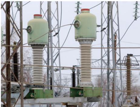
(a) Current Transformer(CT)
