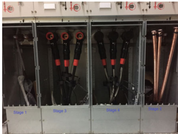
(b) Cable Termination
