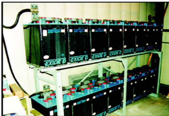
Fig. 4.5 Battery and battery charger
