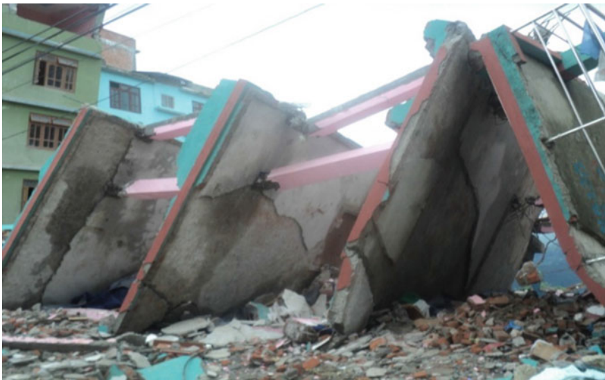
Fig. 20.6 Earthquake devastation in Charikot
