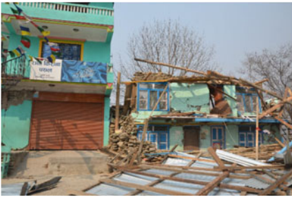
Damaged building by 4-25 Earthquake (Photo by Jianqiang Zhang)
