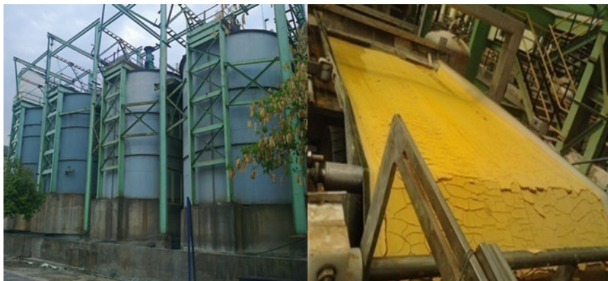
Fig. 7 Mechanically agitated tanks and horizontal belt filter at Turamdih Plant
