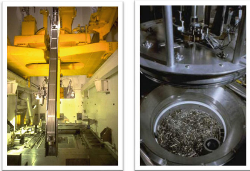
Fig. 2 Fuel assembly cutting unit and compacting unit—La Hague
