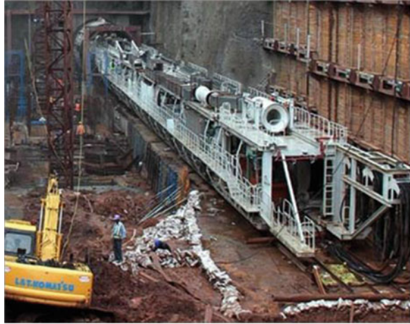
Fig. 12.9 Tunnel boring machine which is assembled for a length of 96 m begins the tunneling work (Ref: http://www.delhimetrorail.com/whatnew_details.aspx?id=c4kjd1nWTgMlld )
