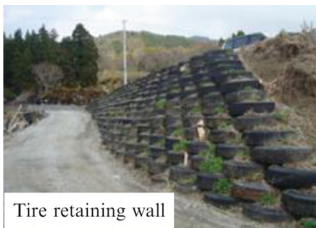
Fig. 9.1 Tire retaining wall in Okirai, Iwate Prefecture (picture taken after the disaster)
