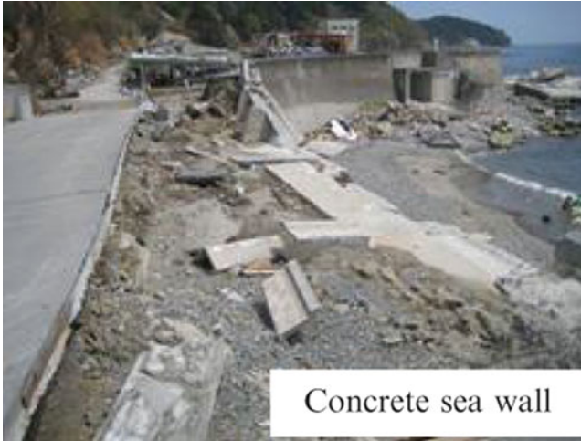
Fig. 9.2 Collapsed seawall in Okirai, Iwate Prefecture
