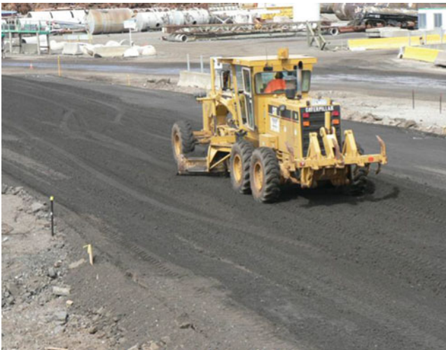
Fig. 1.2 Laying of the base layer at one of the sections including a fraction of FRG (Arulrajah et al. 2013a)
