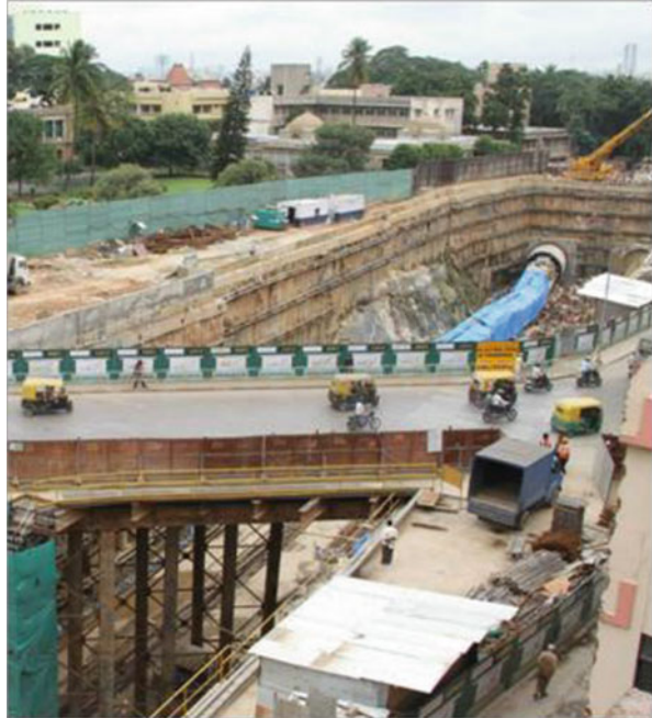
Fig. 12.6 Underground twin tunnel TBM construction near Kalasipalyam, Bangalore. (a) North-south alignment, (b) east-west alignment
