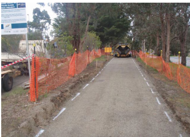
Fig. 1.4 A sections of shared path after field compaction of base layer (Arulrajah et al. 2013b)
