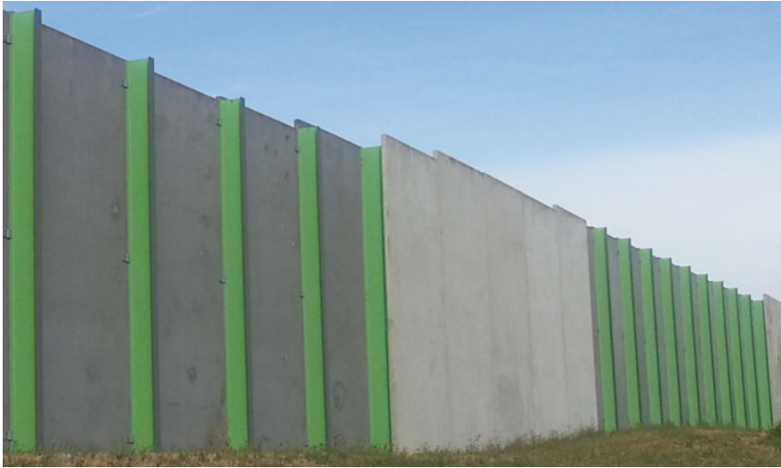
Fig. 3 Highway noise barrier that has both wood panels and light weight concrete panels
