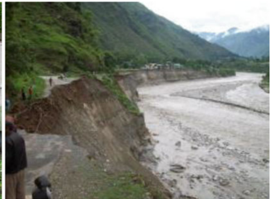
Damaged Roads in Uttarakhand Flash Floods
