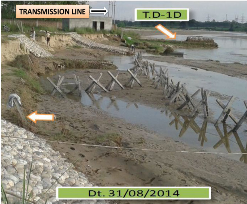
Fig. 15.28 Implementation of RCC jack jetty to inhibit further erosion between T.D-1 and T.D-1D
