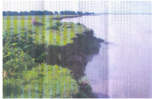
Fig. 14.10 Erosion on right bank u/s of Mahananda bridge
