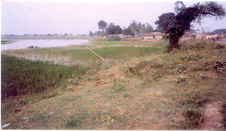
Fig. 14.13 Erosion on left bank of Bagmati River damaging the habitats on outer bank of 90° Bend u/s of Bagmati bridge
