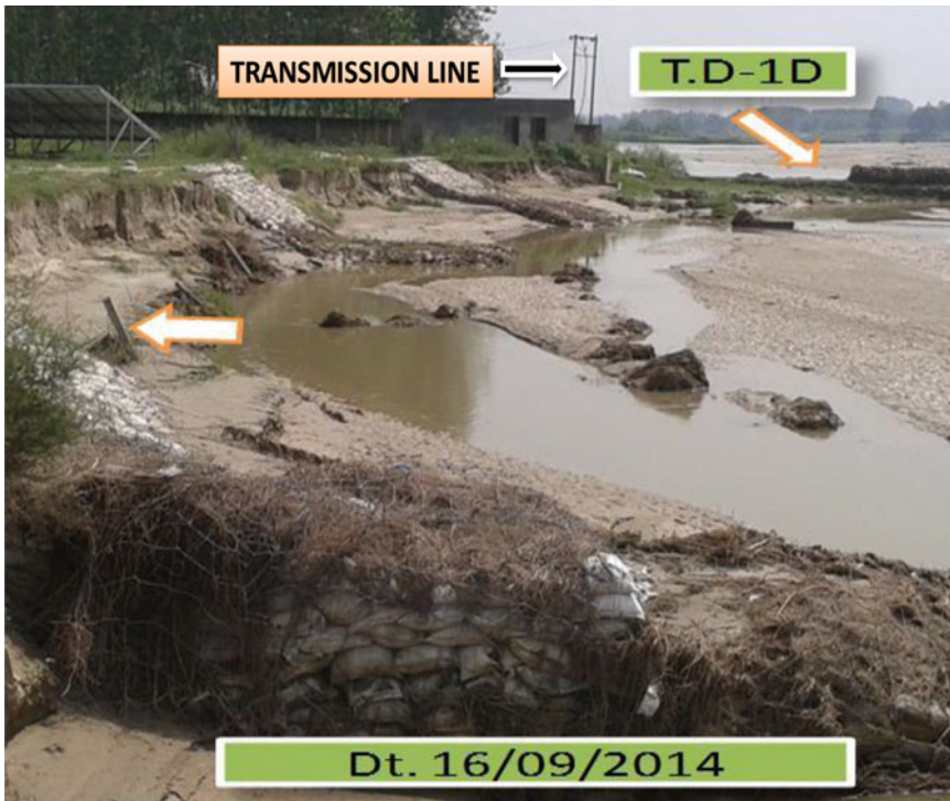
Fig. 15.29 Siltation, inhibition of bank erosion between T.D-1 and T.D-1D and protection of transmission line
