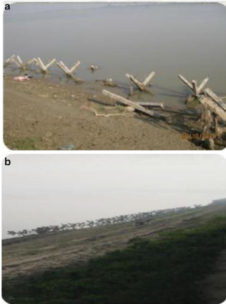
Fig. 15.13 Silting of banks with the RCC jack jetty (a) view of jacks along banks of channel (b) looking down to the channel banks
