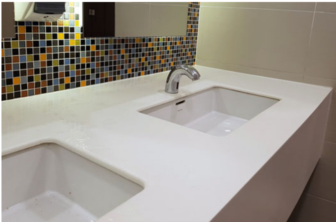
Fig. 8.2 Photo showing a sensor controlled water tap
