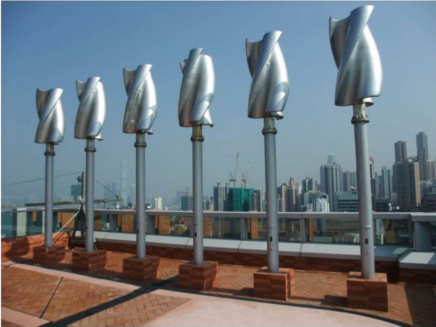
Fig. 7.4 Photo of vertical axis wind turbines installed on top of a building at the Hong Kong University campus
