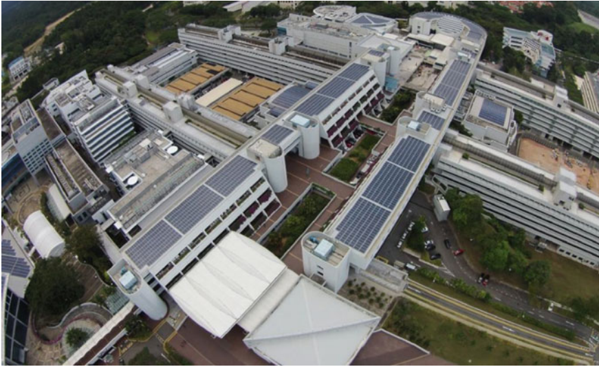
Fig. 7.1 Photo of solar panels installed on the rooftop of the NTU campus buildings in Singapore
