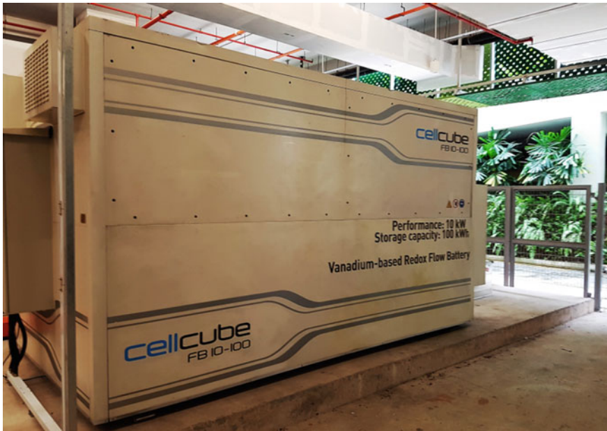
Fig. 7.6 Photo of a Vanadium Redox-flow battery (VRB) installed in the basement of building in Singapore
