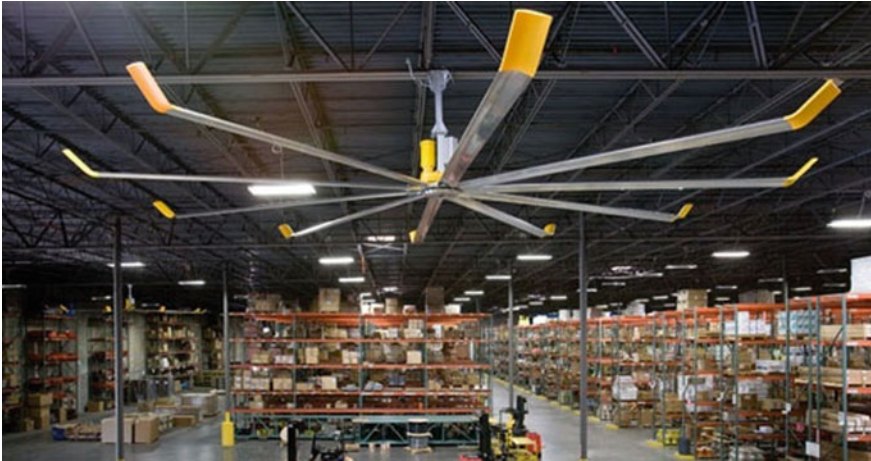
Fig. 5.11 Photo of HVLS fan installed in an industrial workshop space (Kestrel Services)
