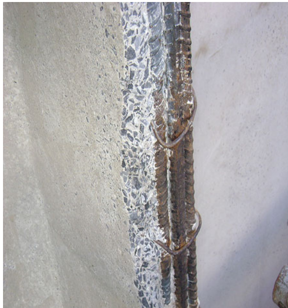
Fig. 6 Reinforcement concentration, 4 rebar 20 mm diameter and low reinforcement coverings (6 mm) of concrete. The structure is already attacked by hydrochloric acid vapors. Source Authors, 2013
