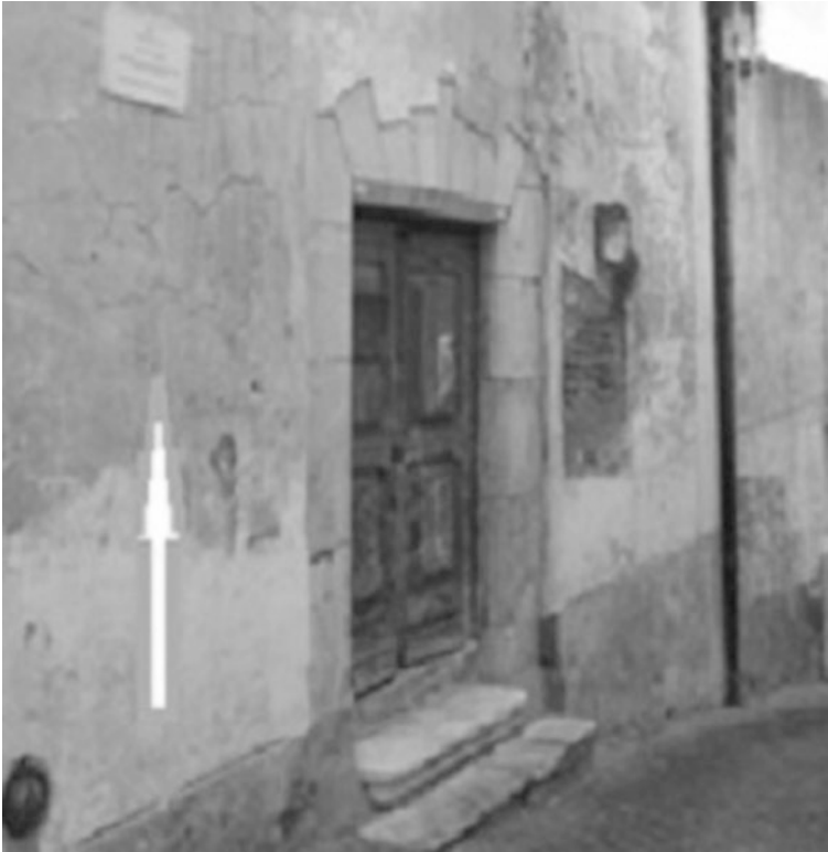
Fig. 8 Diffuse cracking of the coating on the main facade
