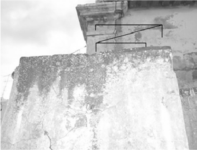
Fig. 10 Possible interventions with stapling, inserted in the wall and in the stonework
