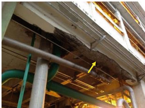
Fig. 28 Beam with virtually no frames
