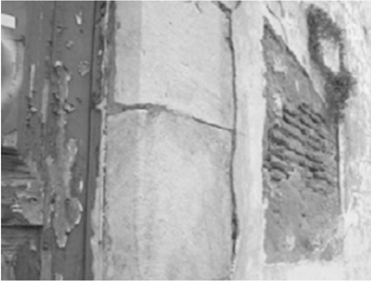
Fig. 7 Revetment overlaps the stone with invasive vegetation
