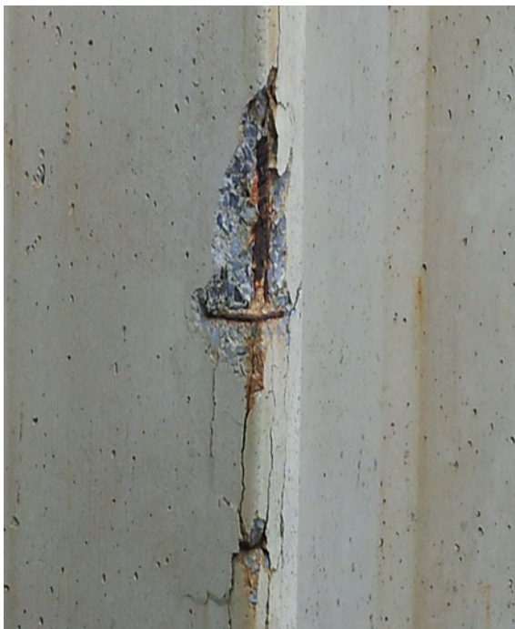
Fig. 4 Cracking and spalling, parallel to the reinforcement
