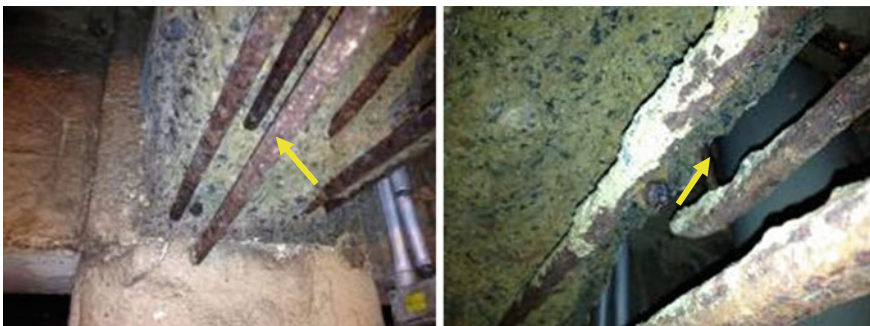
Fig. 26 Stress corrosion cracking reinforcement
