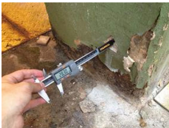
Fig. 31 Pilar with high carbonation depth along the floor (M)
