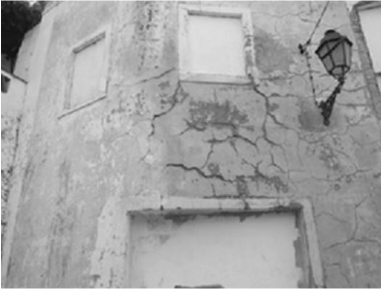
Fig. 11 Cracks under the sill of the window and in the lintel
