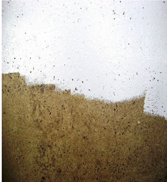
Fig. 14 Application of epoxy varnish sealer and application of intermediate coat in epoxy two-component polyamide cured. Source Authors, 2013
