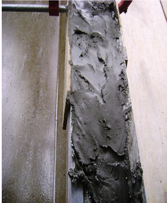
Fig. 13 Application of structural cementitious mortar for repairs up to 7 cm deeper. Source Authors, 2013
