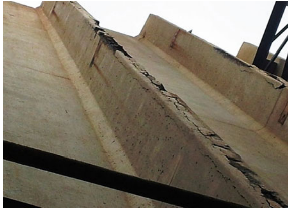
Fig. 2 Pathologies presented by fence panels. Source Authors, 2013
