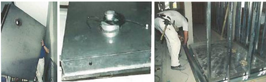
Fig. 7 Left Floor element seen from the top, Middle floor gully at bottom plate and Right installation of walls to the floor. Pictures from Danish Ministry of Housing and Urban Affairs (2001b)
