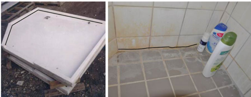
Fig. 15 Left Fibre reinforced bottom plate with a plinth marked with a black line . Right The black line indicates the crack, which was found on different walls in the bathroom above and below the apartment on the picture. Left Picture from Danish Ministry of Housing, Urban and Rural Affairs (1999b)
