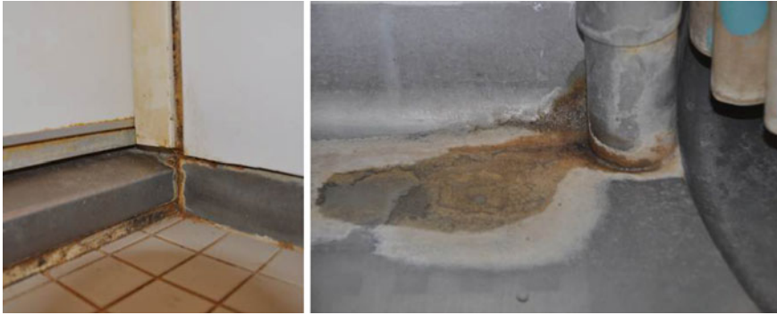
Fig. 16 Left Bathroom #4, the corner of the door, wall and floor assembly where the rusty red colour is anticipated to be mould growth as it is the same colour as seen on the silicone sealant. Right Rusty red colour at each corner at the interface of the shower unit and floor, see also Fig. 9
