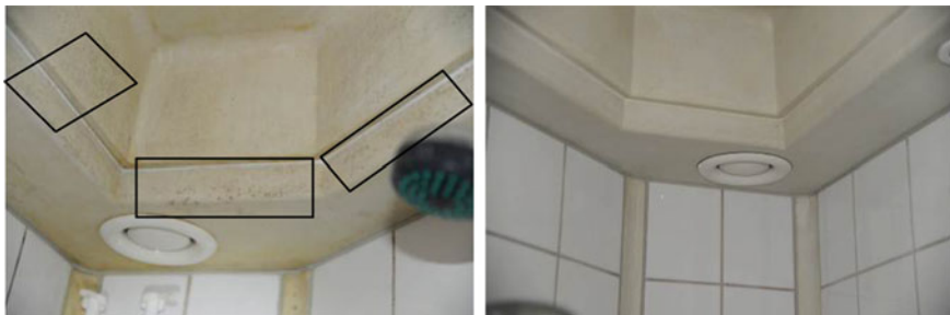
Fig. 17 Two bathrooms connected to the same ventilation exhaust, but where the one ( left ) has a low rate of extraction and dark stains in the ceiling, whereas the other ( right ) has a high rate of extraction and no dark stains in the ceiling
