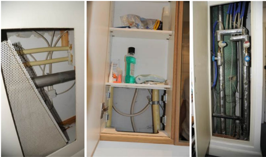
Fig. 18 Left Access to installations through a hatch in the ceiling. Middle A small cabinet gives access to the installations. Right Access to the installations through a door in the bedroom
