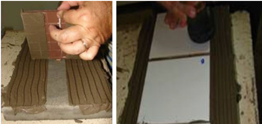
Fig. 2 Placement of the ceramic tiles with central defect
