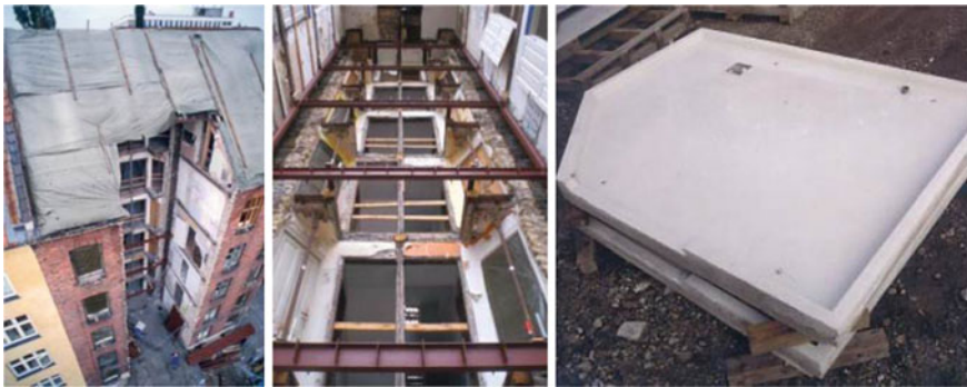
Fig. 12 Left Opening in the building after demolishing kitchen, toilet and floor division. Middle Inner frame of new floor structure for carrying the bathroom and new kitchen. Right Fibre reinforced floor element with a plinth. Pictures from Danish Business and Housing Authority (2004a), Danish Ministry of Housing, Urban and Rural Affairs (1999b)
