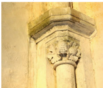
Ice formation on walls (Pöide Church)
