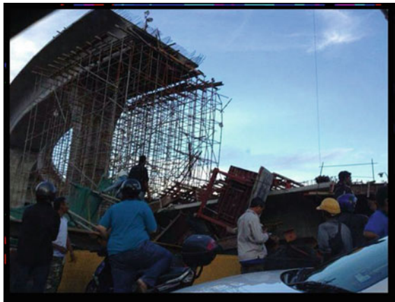
Fig. 1 30 m wide ramp of the bridge under construction collapsed (NST, 2013)
