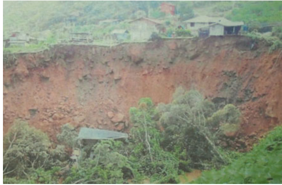
Fig. 2 Landslide triggered by earthquake on 5th June 2015 in Kundasang (source from The Star, Thursday 18th June 2015)
