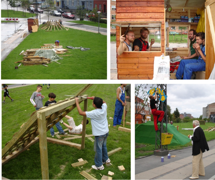
Figure 2. 2.1. The Hill. Beginning the process of construction. 2.2. The artists of Parfyme having lunch inside the mobile site-shed. 2.3. Constructing soccer-goals. 2.4. Dialogue with passers-by. Photos: Parfyme
