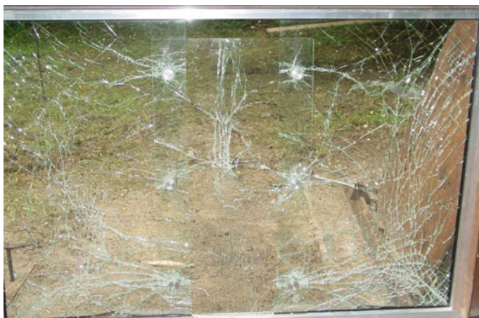
Fig. 18.13 Damage to the cash desk protective window following the third application of the air shock wave
