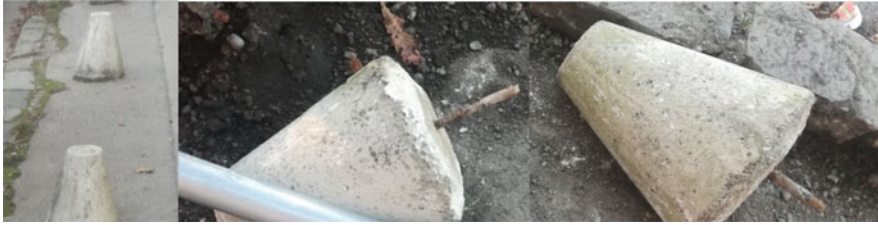
Fig. 9.3 Designed physical barriers without no resistance capacity
