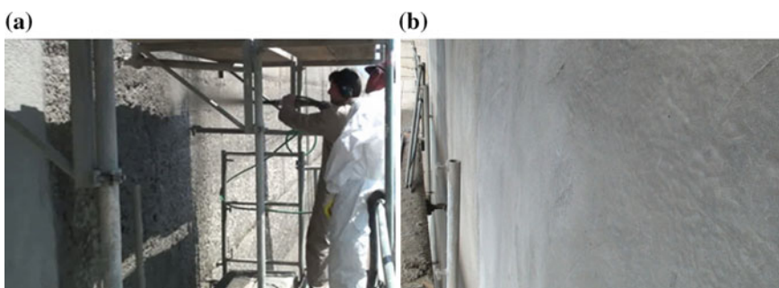
Fig. 1.11 a Application of SHCC containing SAP as repair material for spraying ( \times 3 ), b condition of the surface after completion of the repair work (courtesy of Professor Viktor Mechtcherine, TU Dresden)
