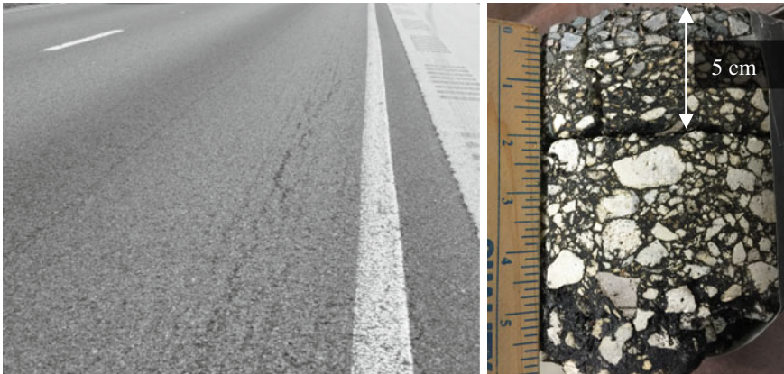
Fig. 1 Presence of near-surface longitudinal cracking concurrent with interface debonding in I-10 interstate highway (Duval County, Florida)
