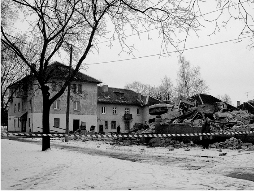
Fig. 5.3 Demolition of an abandoned building at 1 Vahtra Street (Photo by Anu Printsman)
