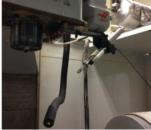
Fig. 24.2 The pre-cooling cryogenic setup: shown is the nozzle at the end of the piping system from accumulator to the workpiece fixtured on HAAS vertical machining center
