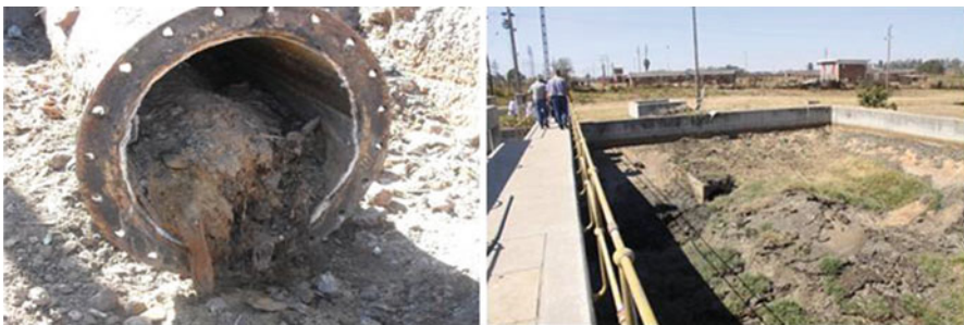
Fig. 4.2 High levels of sand in sewers ( left ) can cause downstream problems at sewage treatment plants ( right ) (Photographs: City of Harare)
