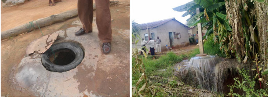
Fig. 4.5 Use of unprotected shallow wells ( left ) and protracted sewer overflows ( right ) became very common, especially in high density suburbs, during the 2008 cholera outbreak in Zimbabwe (Photographs: I. Nhapi)
