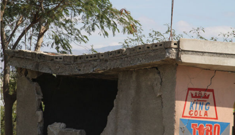
Fig. 9.4 Example of heavy slab built primarily for resisting gravity loads and hurricanes
