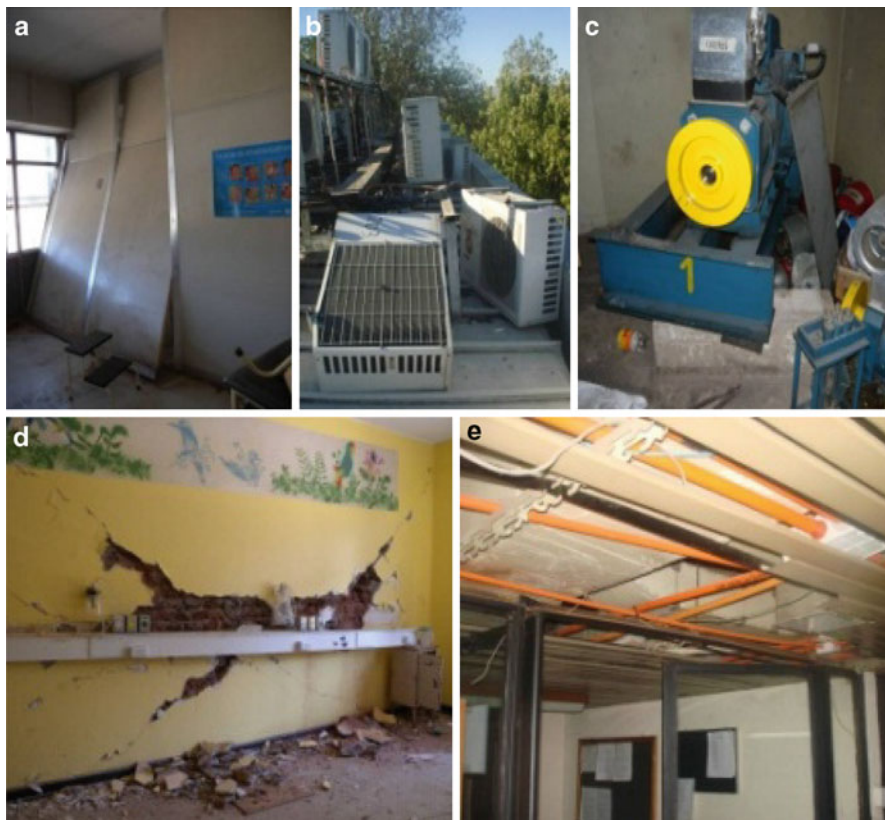
Fig. 11.4 Examples of nonstructural damage: (a) Damage to floating partition walls, (b) Damage to HVAC equipment, (c) Damage to driving system, (d) Damage to rigidly connected partition walls, and (e) Damage to suspended ceilings
