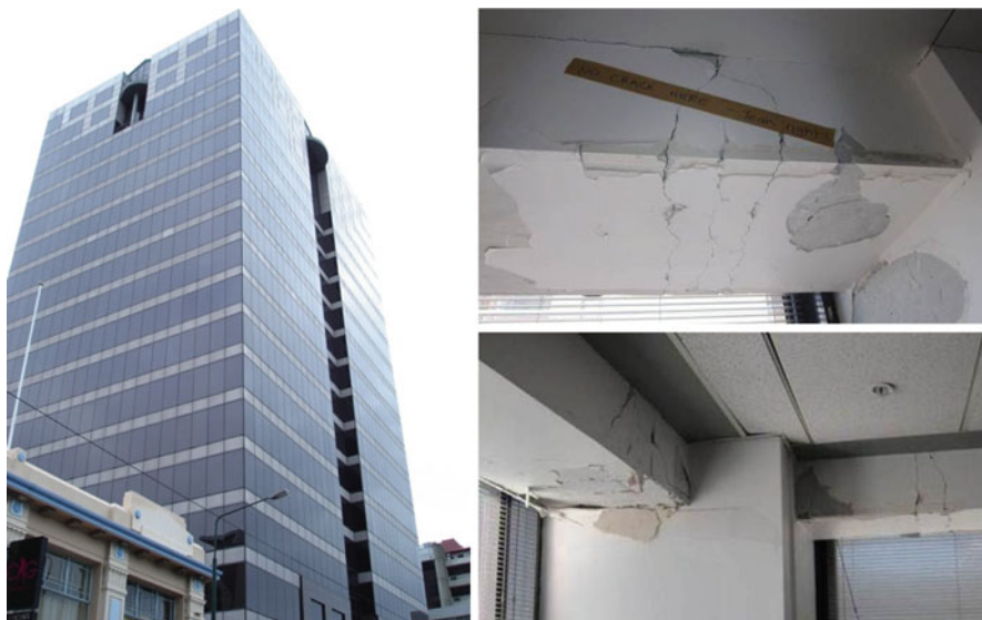
Fig. 12.3 Beam cracking in a 22-story RC moment frame (precast emulating cast-in-place) scheduled to be demolished
