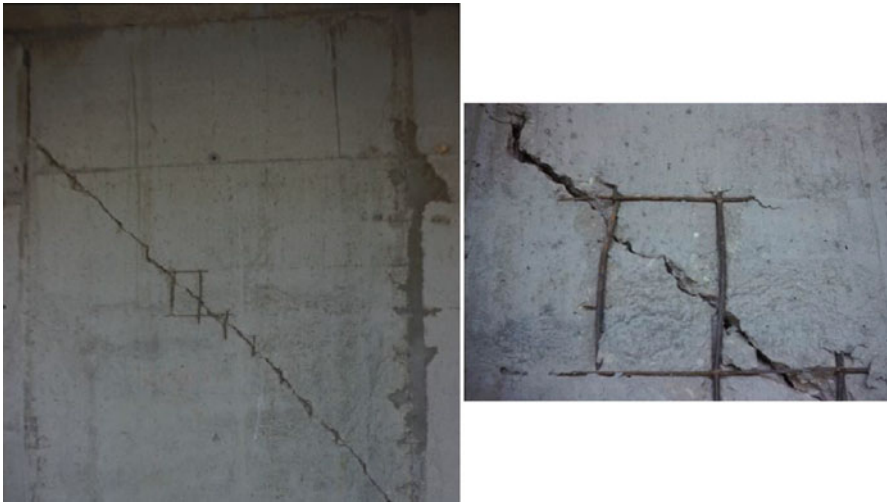
Fig. 24.3 A pier in a coupled wall damaged during the 1979 Montenegro earthquake
