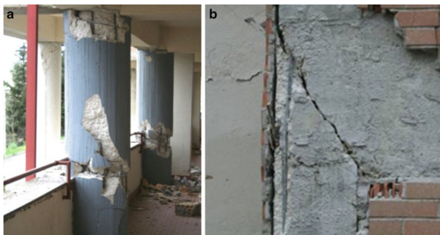
Fig. 10.6 (a) Shear failure of column adjacent to partial infilling panels; (b) diagonal cracking failure in concrete joint panel (Ricci et al. 2011a)
