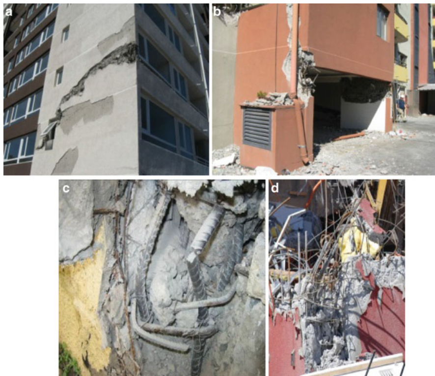
Fig. 11.6 (a) Shear Failure Example in a new 25 story building. (b) Compression-tension failure in elements supporting walls. (c) Fractured of longitudinal reinforcement after buckling. (d) Lap-splice failure
