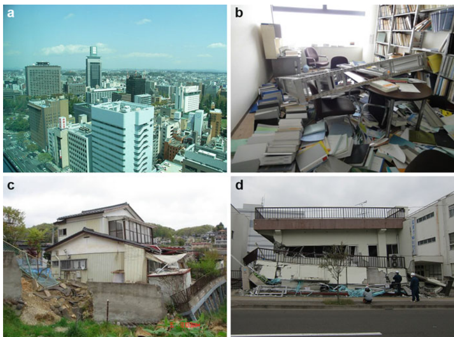
Fig. 8.8 Response of buildings in Sendai area to the earthquake (a) Downtown Sendai after event (b) Nonstructural damage (c) Landslide damage (d) Shear failure and collapse of two-story RC building
