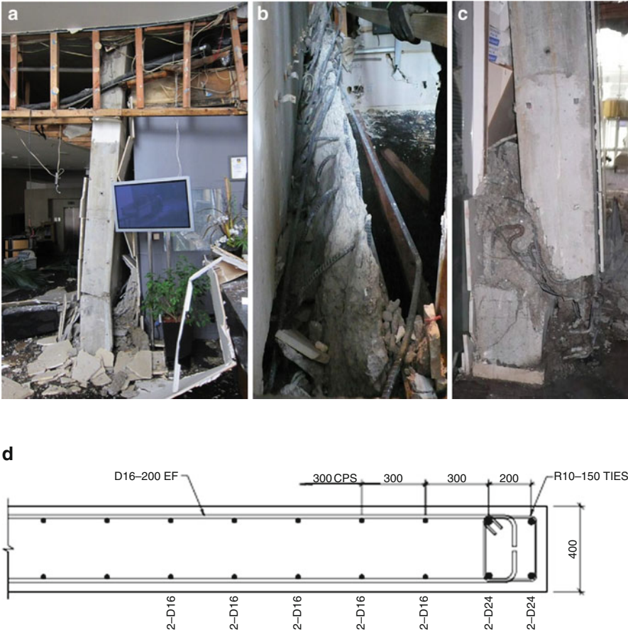
Fig. 12.7 Crushing and out-of-plane movement of shear wall in 22-story Hotel Grand Chancellor: (a) Lobby wall; (b) close up of failure at splice; (c) out-of-plane movement of wall; (d) reinforcement details (Photos (b) and (c) from Dunning and Thornton 2011)
