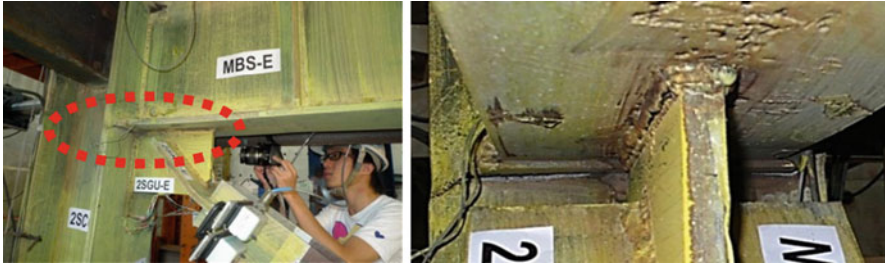
Fig. 17.7 Fracture of inner flange of the 2nd story south column top near the gusset at the earthquake time 5.67 s
