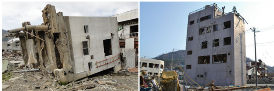
Fig. 8.10 Overturned versus standing RC buildings after the tsunami
