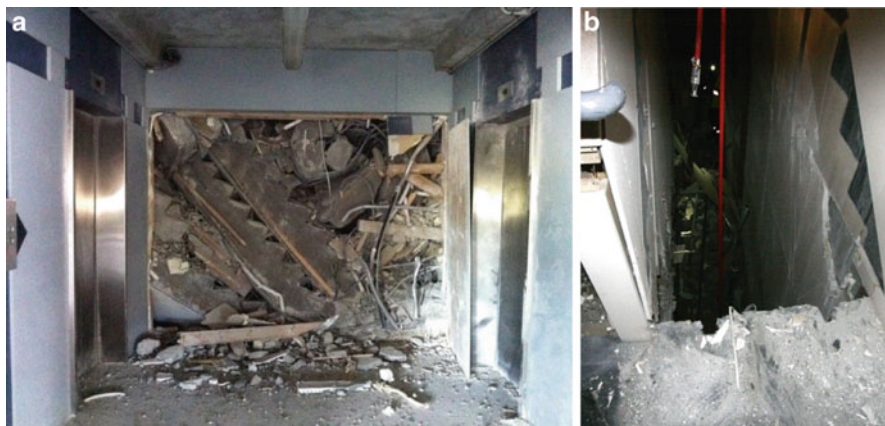
Fig. 12.8 Collapse of precast stairs: (a) Forsyth Barr building; (b) hotel Grand Chancellor
