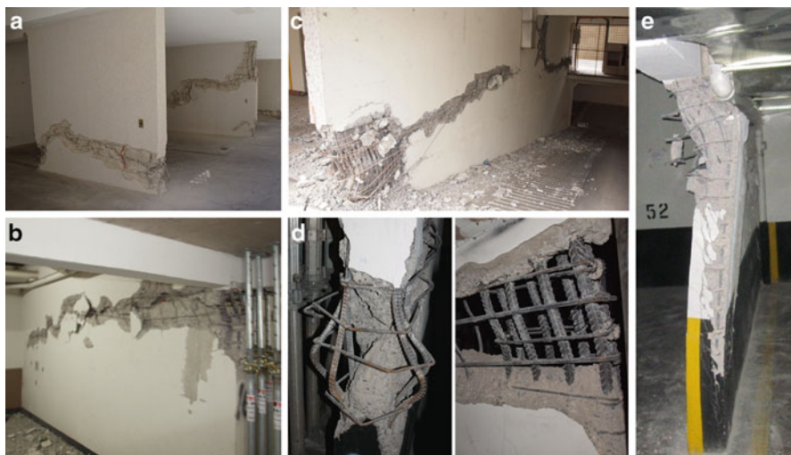
Fig. 30.1 Typical wall damage in Chile earthquake. (a) Vina del Mar. (b) Santiago. (c) Concepcion. (d) Boundary zone details. (e) Wall lateral instability
