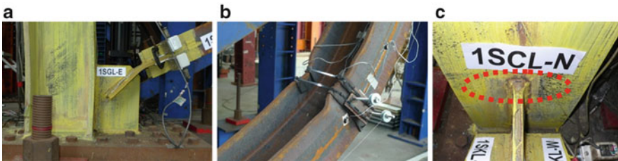
Fig. 17.8 (a) The deformed condition of the knife plate, (b) local buckling of the 1st-story south brace, and (c) weld crack at the gusset edge
