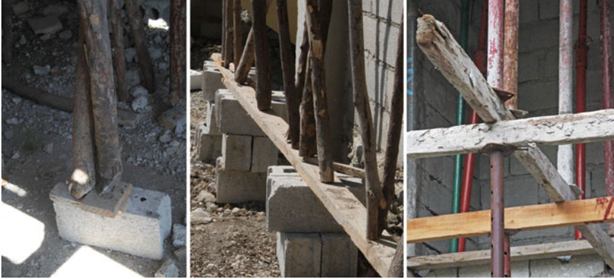
Fig. 9.5 Examples of poor construction practice even for resisting gravity loads
