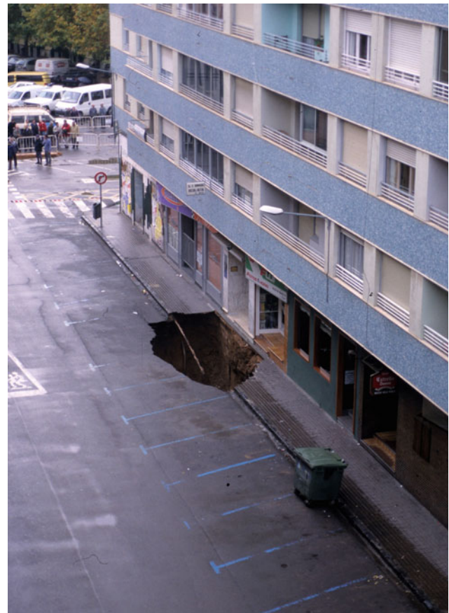
Fig. 9.11 Collapse sinkhole occurred catastrophically in 10 November 2003 next to and beneath the Blue House . Photograph taken in the morning of November 10
