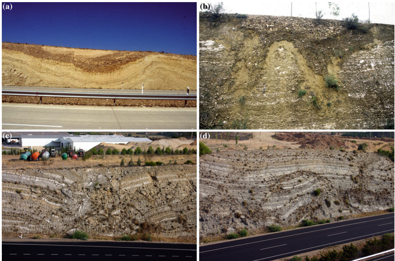
Fig. 9.8 Dissolution and subsidence structures exposed in cuttings of the Madrid–Zaragoza highway (A–2) along the southern margin of Jalón Valley. a Sagging in terrace deposits related to the dissolutional lowering of the evaporite rockhead. Note the marly karstic residue between the bedrock and the cover. b Dissolutional conduits filled with alluvium derived from the overlying terrace deposits. c Sagging and
