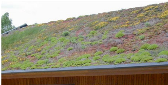
Fig. 12.8 Roof garden containing a range of Sedum pp. (Photograph courtesy of A. Bettin)
