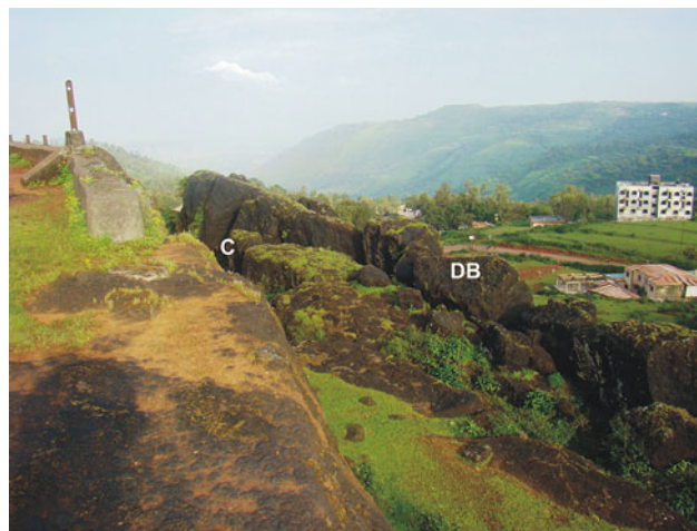
Fig. 6 Evidence of mechanical disintegration of the indurated crust. Note the presence of clefts C and partially to completely detached blocks of laterites DB at the margins of the crust. Location indicated by B in Fig. 3
