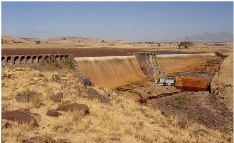
Fig. 1.6 The Aba Samule Reservoir on the Akaki River, south of Addis Ababa ( 8^{\circ}47'15''\text{N} – 38^{\circ}42'18''\text{E} ). The dam was constructed in 1939 but a few decades later it was completely filled with sediment
