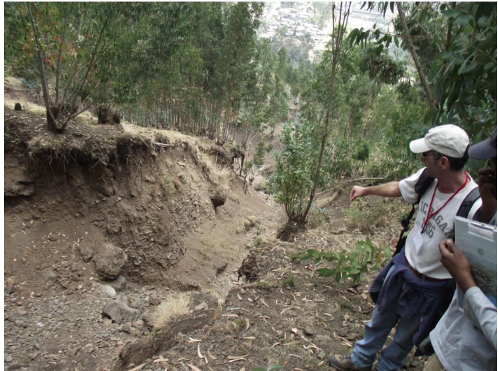
Fig. 20.18 Trench of a deep-reaching translational debris slide at Dese
