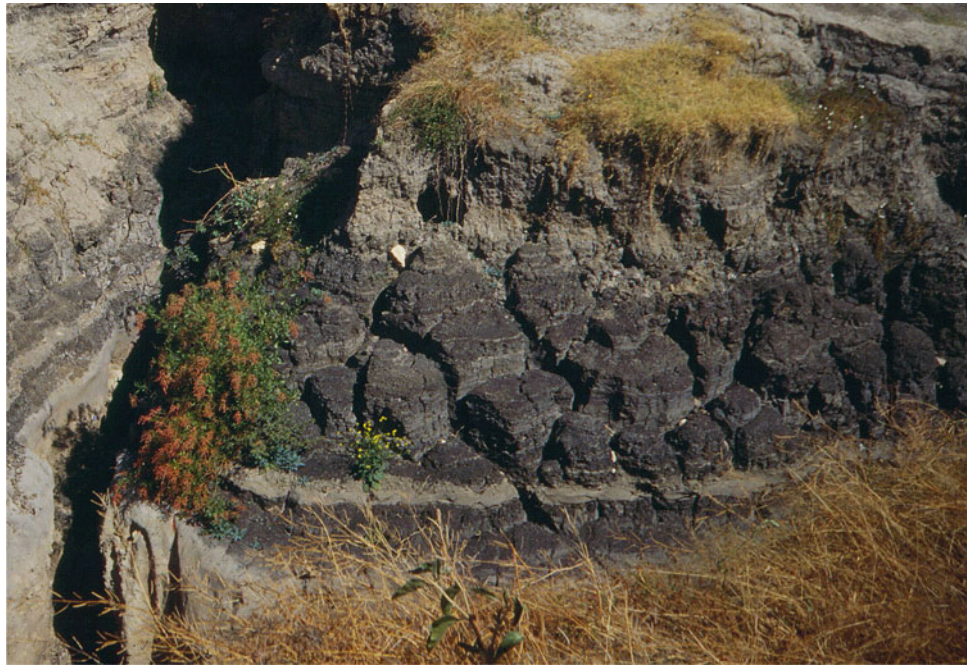
Fig. 11.9 Desiccation cracks in the lower part of the Mai Makden tufa dam backfill
