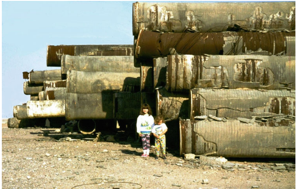
Fig. 13.1 Water pipeline ruined by salt attack between Rössing and Swakopmund
