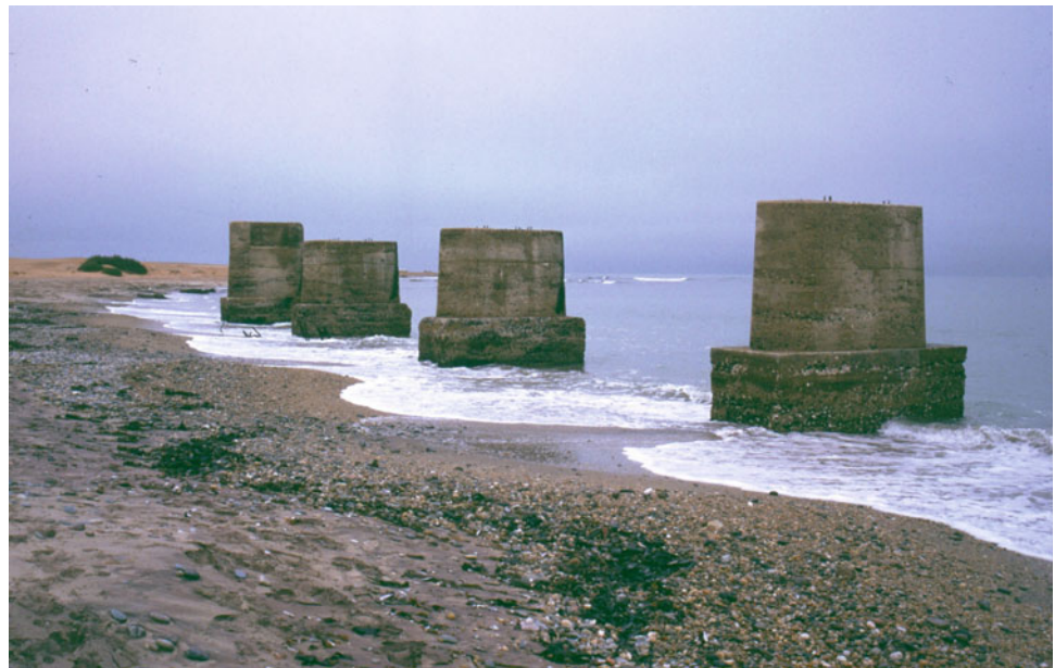
Fig. 1.10 The remains of the same bridge at the mouth of the Swakop which was demolished by a flood in 1931
