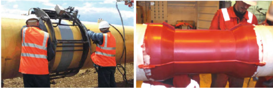
Fig. 14.17 Application of a field coated joint, as exemplified by a the flame-sprayed, and b the heat shrink sleeve, methods [69]
