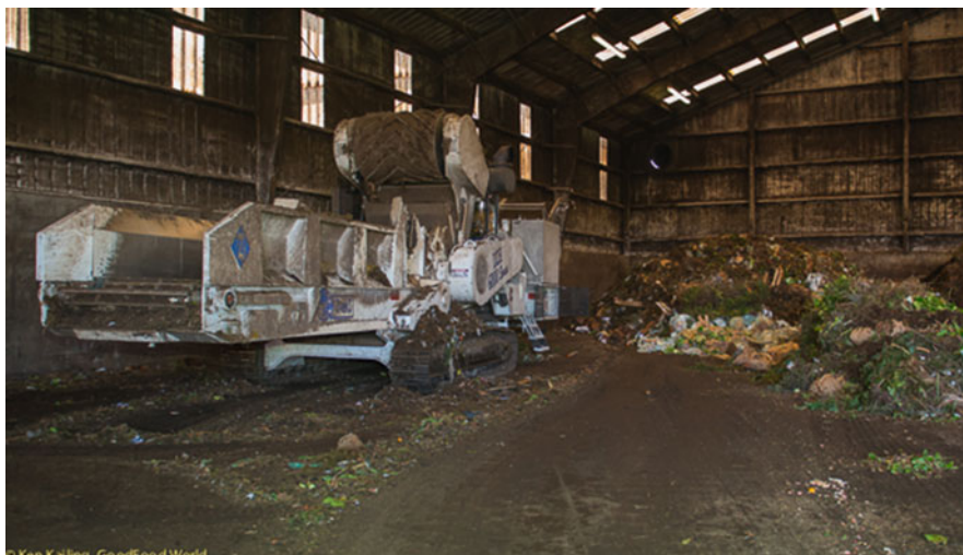
Fig. 3 A grinder inside the receiving facility. The grinder grinds feedstocks to fixed particle sizes allowing for rapid composting
