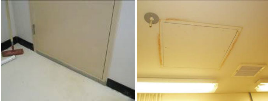
Fig. 11 Door sweeps and blocked escape routes
