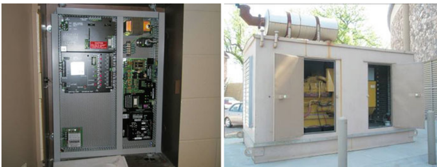
Fig. 12 Alarm system and backup generator
