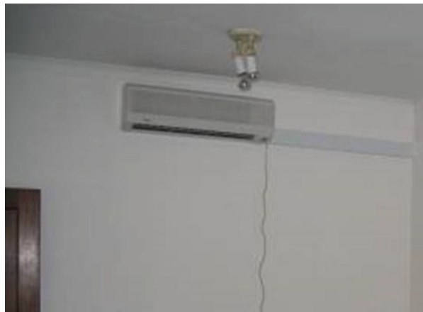
Fig. 4 Wall air-condition unit
