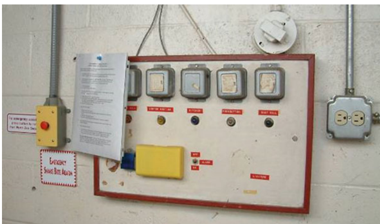
Fig. 13 Alarm system mounted on a wall
