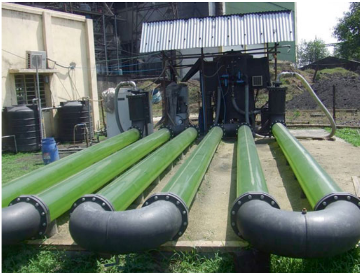
Fig. 4 A tubular photobioreactor used for growing microalgae in a power plant (image courtesy © D. Sahoo)
