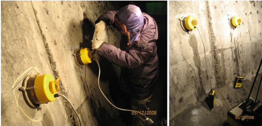
Fig. 8.41 Testing concrete quality with PERMIT in Harbin-Dalian railway project by Tsinghua University
