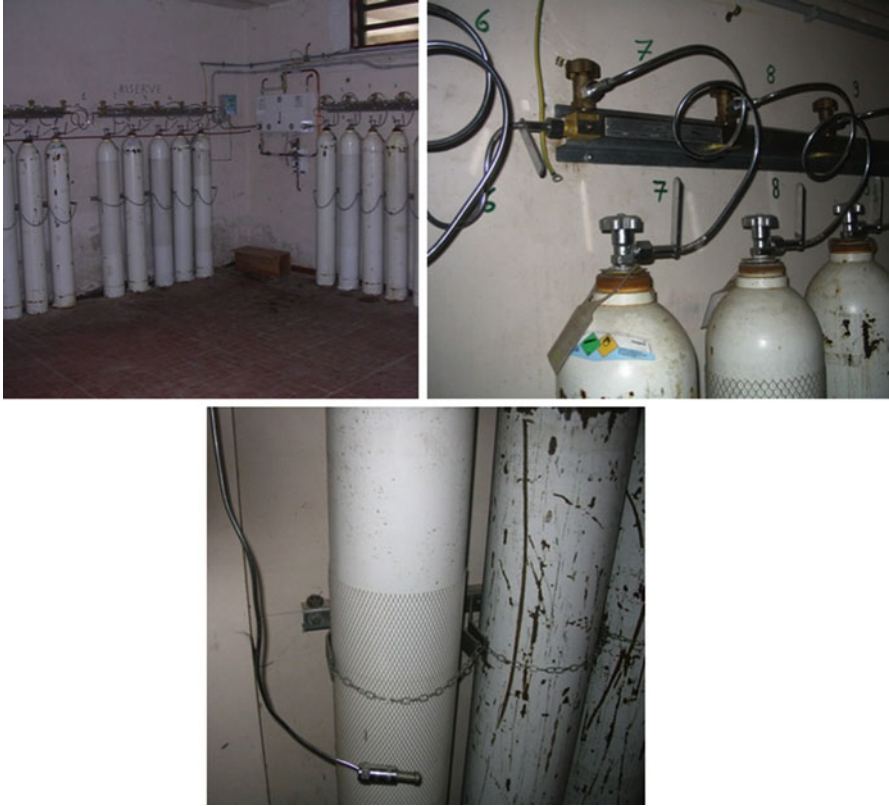
Fig. 12.10 Example of oxygen cylinders – detail of anchorage
