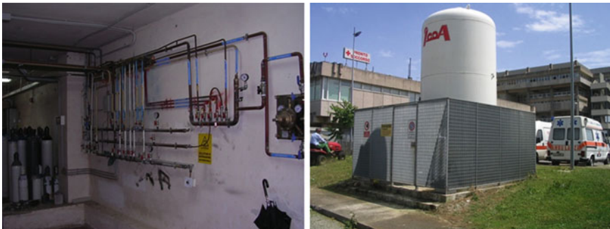
Fig. 12.11 Examples for distribution lines ( left ) and for oxygen bottle tank ( right )
