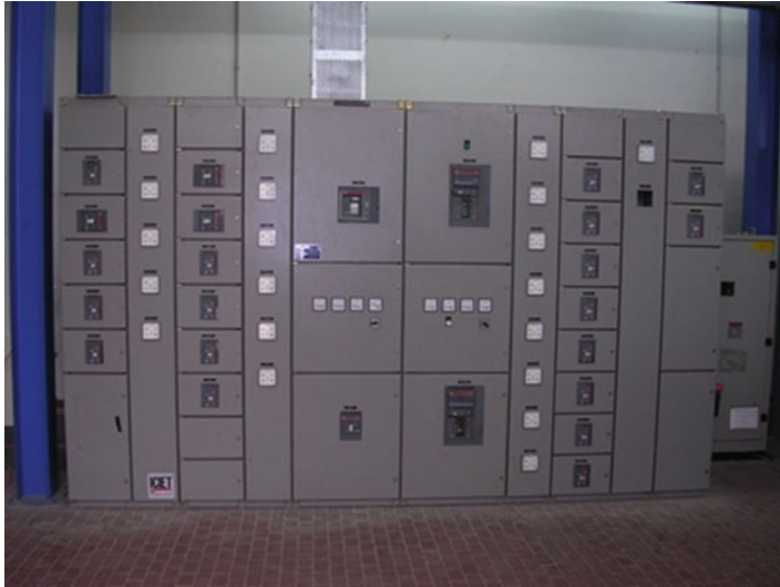
Fig. 12.16 Example of general switchboard panel
