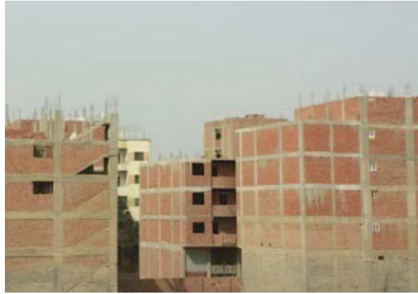
Fig. 5 The typical type of the slums buildings, permanent with reinforced concrete skeleton and bricks, note the lack of windows as inner rooms depend on light wells
