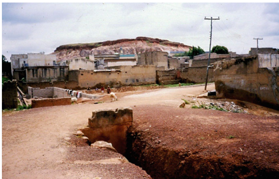
Fig. 4 Residual of laterite duricrusted African surface with underlying deep weathering. Kano, Northern Nigeria
