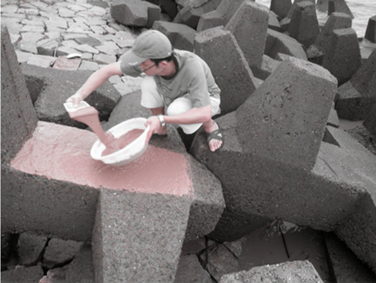
Fig. 8.6 Application of an alkali-activated binder coating to marine concrete elements in China (Photograph courtesy of Z. Zhang, University of Southern Queensland)
