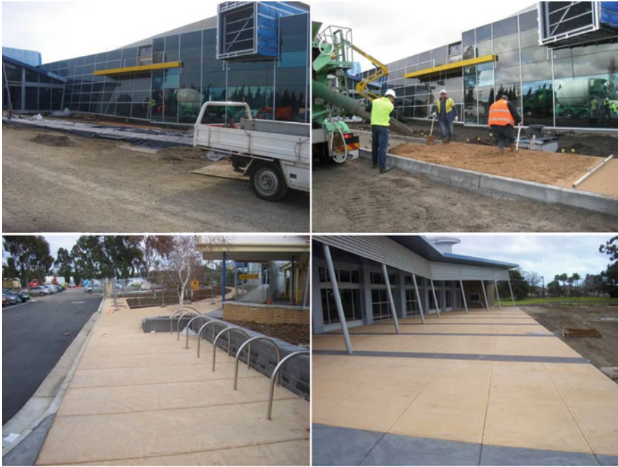
Fig. 11.19 E-Crete pavement and in situ works for Thomastown Recreation and Aquatic Centre, Melbourne, Australia
