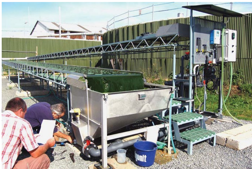
Fig. 7 Pilot-scale photobioreactor for thin-layer cultivation of Chlorella algae in a dairy farm (1,200 pcs of dairy cattle) at Dublovice, Czech Republic. After combustion of an anaerobically generated \text{CH}_4 flue gas is used as a source of \text{CO}_2 for algal photosynthesis. A modified liquid fraction of anaerobically digested manure can serve as an additional source of nutrients. (Photograph by J. Langová, BCS Engineering)
