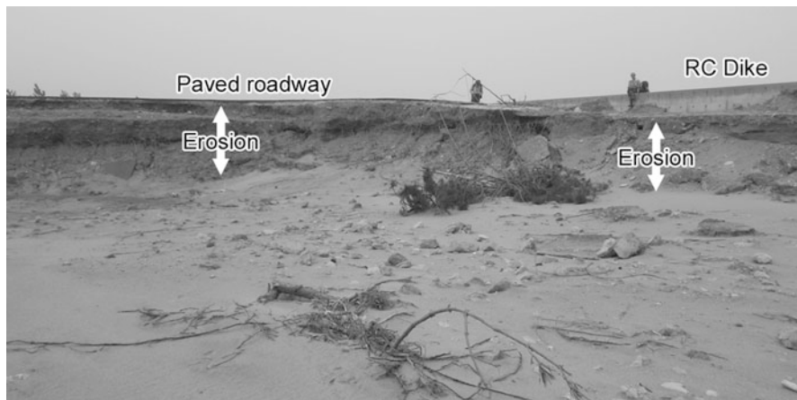
Fig. 4.2 Erosion at the back of the reinforced concrete dike at Point 1 in Fig. 4.1b
