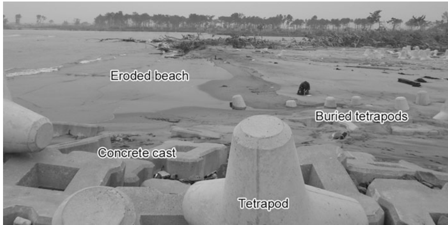
Fig. 4.3 Collapsed RC dike and erosion of the sand bar at Point 2 in Fig. 4.1b. Concrete casts that comprised the dike were scattered and buried by sand
