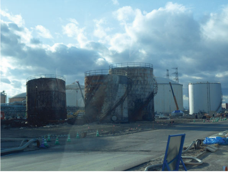
Fig. 15.7 Fires and threats to surrounding facilities: Case of a Japanese refinery damaged by fires that occurred during the sequence earthquake-tsunami Tohoku, March 2011 (Author's pictures)
