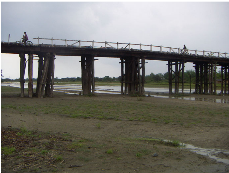
Photo 18.1 A timber bridge, use of wooden pillars as columns, north of Brahmaputra, Eastern Assam (Photo S. R. Jog)
