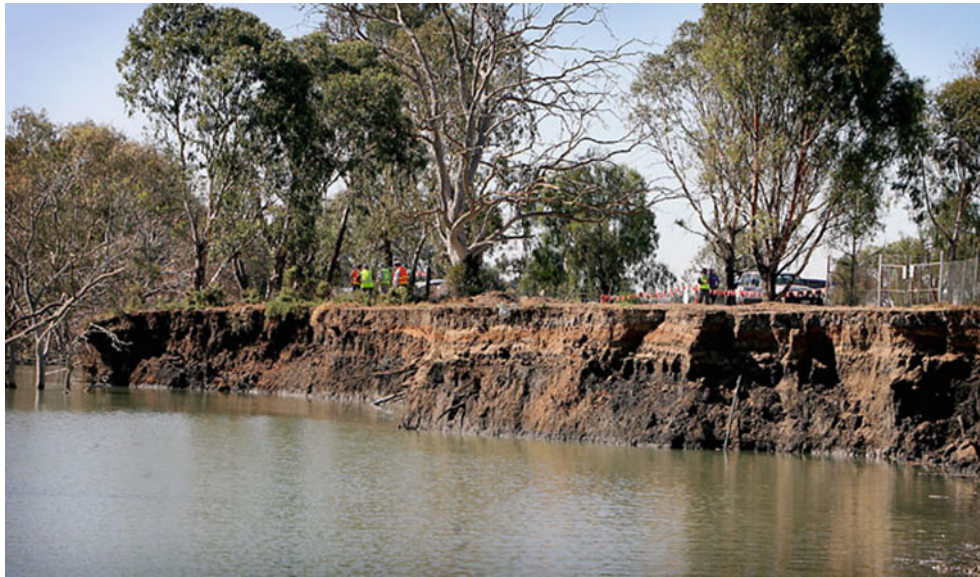
Fig. 9 Collapse of Long Island river bank (near Murray Bridge) in March 2009 (Photo courtesy of News Limited, Australia)
