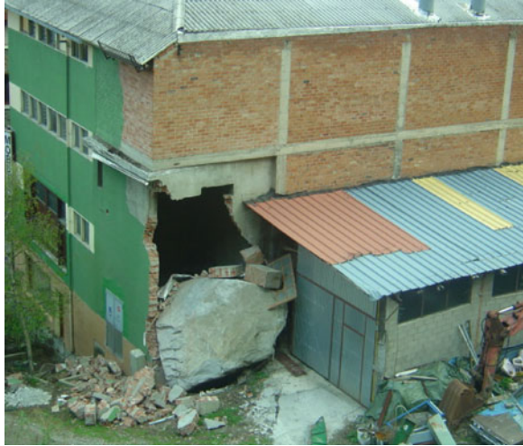
Fig. 6.5 Nonstructural damage at a workshop in Santa Coloma (Principality of Andorra) due to rockfall in April, 2008. No further damage was produced because none of the columns were impacted and broken by the block
