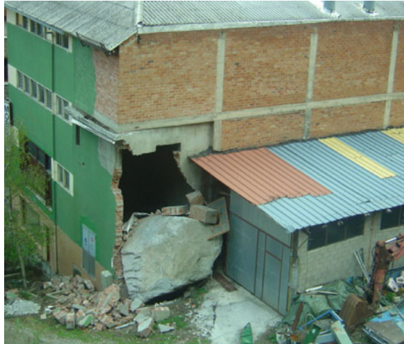
Fig. 6.5 Nonstructural damage at a workshop in Santa Coloma (Principality of Andorra) due to rockfall in April, 2008. No further damage was produced because none of the columns were impacted and broken by the block
