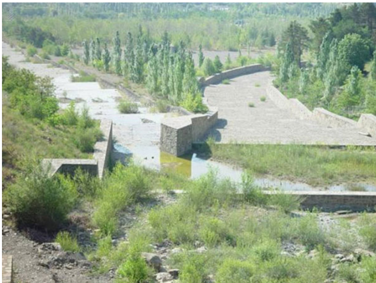
Fig. 11.9 Diversion channel ( right ) at the Biescas debris fan in the Central Pyrenees, Spain. The step-like longitudinal profile will contribute to the energy dissipation of the flow and force debris deposition at the fan apex (© J. Corominas)
