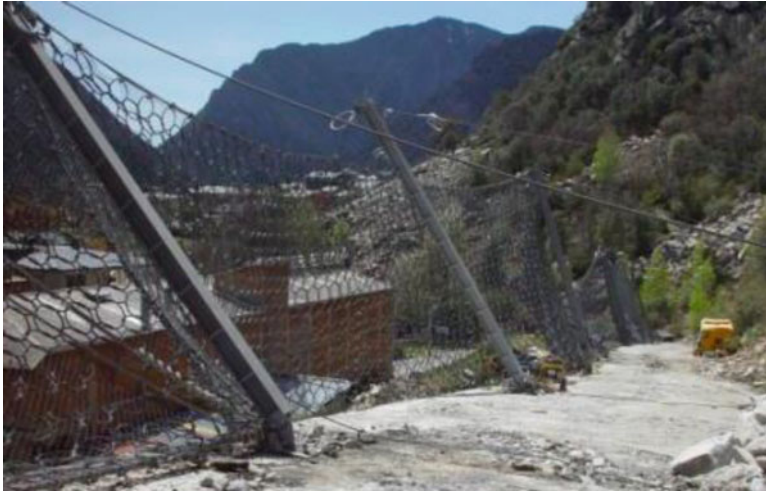
Fig. 11.16 A 2,000 KJ protection fence in Andorra la Vella, Andorra Principality, damaged by a rockfall in April 2008. Replacement of the elements was carried out in a few weeks to immediately restore the protection level of the area (© J. Corominas)
