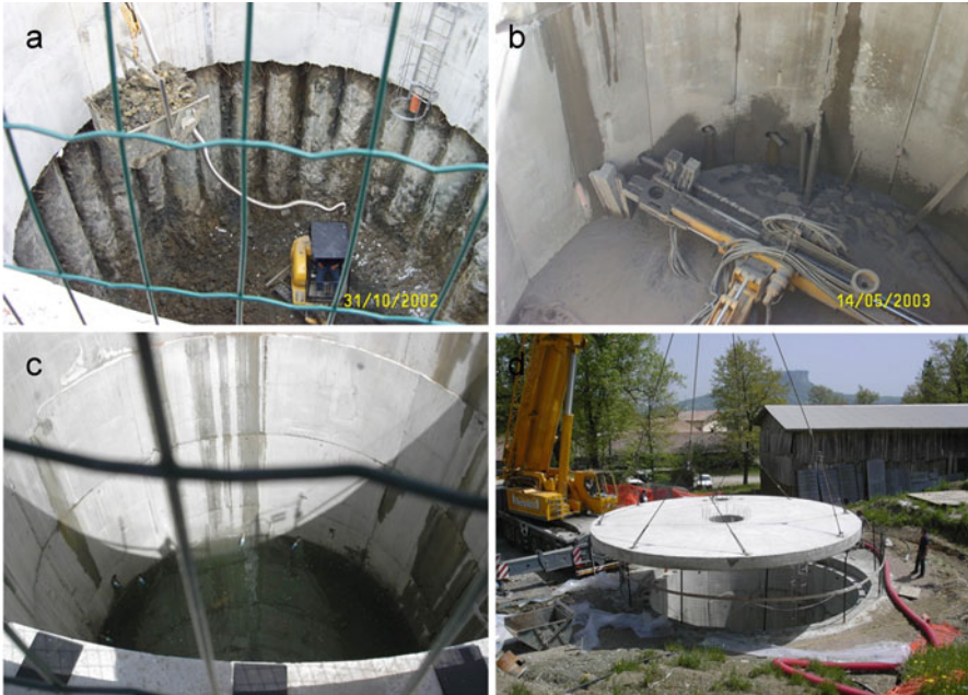
Fig. 11.12 Example of large diameter drainage well (Garfagnolo landslide, northern Apennines, Italy). (a) Excavation inside the circular set of adjacent caisson piles; (b) drilling of radial subhorizontal drains; (c) inner view of the drainage well with water inflow from radial drains; (d) final setup of the drainage system (© G. Truffelli)
