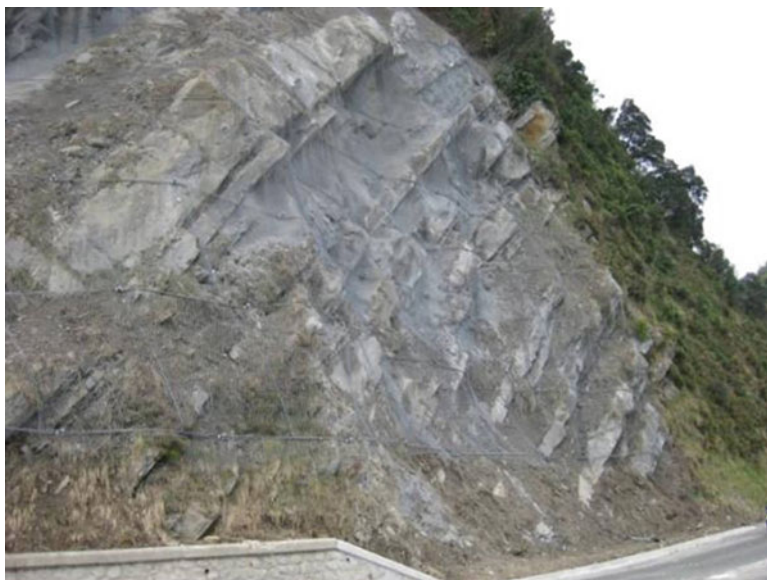
Fig. 11.2 Combined use of rock bolts, shotcrete and wire mesh to prevent rockfalls in the road from Zarautz to Getaria, Basque Country, Northern Spain (© J. Corominas)
