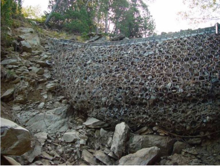
Fig. 11.8 Net at Rumí torrent in Portainé, Eastern Pyrénées. Series of nets are located along the torrent bed, which have been filled with debris (© J. Corominas)
