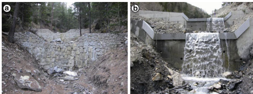
Fig. 10.3 Example of two main types of check dams observed in the Faucon torrent often affected by debris flow events, near Barcelonnette. (a) Photograph of a typical masonry check dam; (b) Photograph of a typical concrete check dam
