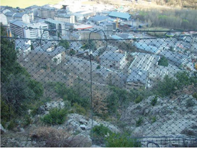
Fig. 11.4 Rockfall fence installed at the Canal de l'Alzina to intercept and/or reduce the velocity of the falling blocks before reaching the bottom of the slope where Santa Coloma neighborhood, Principality of Andorra, is built (© J. Corominas)
