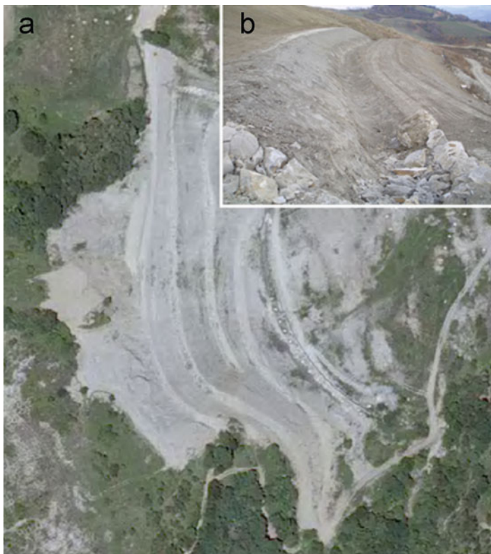
Fig. 11.10 Example of stepped grading of a landslide head scarp zone (Ca’Lita landslide, northern Apennines, Italy). (a) Global view from orthophoto; (b) detail view of benches
