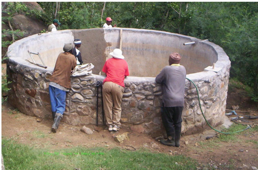
Fig. 8.15 Concrete tank to protect a spring. This project provided jobs and taught skills
